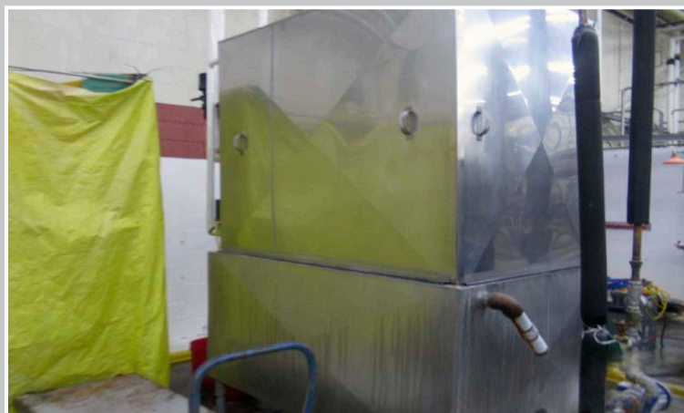
CHESTER JENSON S/S Large Capacity (6) Falling Film Water Chiller
