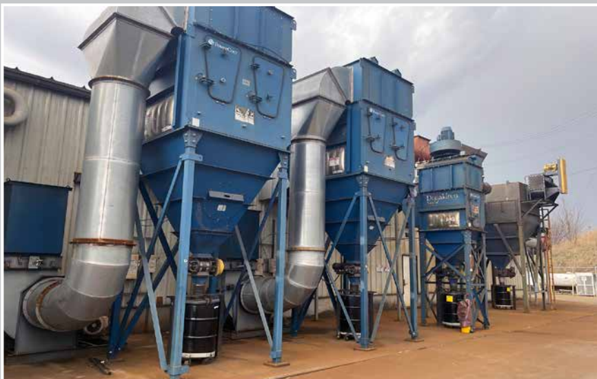
View of Dust Collection System
