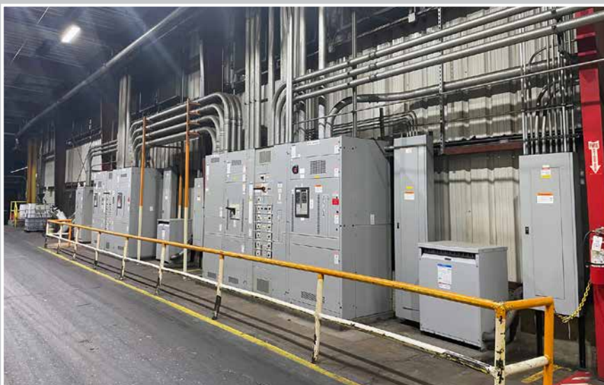
View of Electrical
