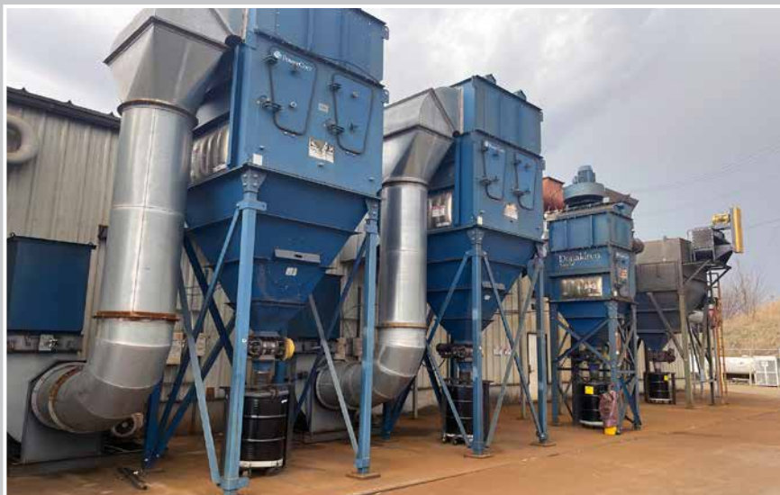
View of Dust Collection System
