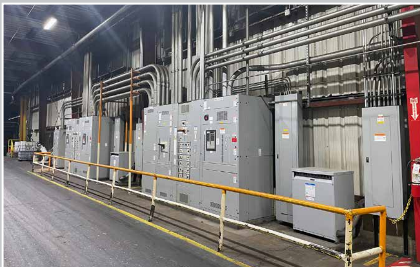
View of Electrical
