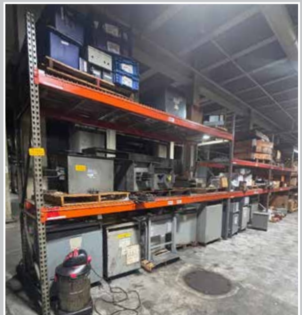
Partial View Electrical Transformers
