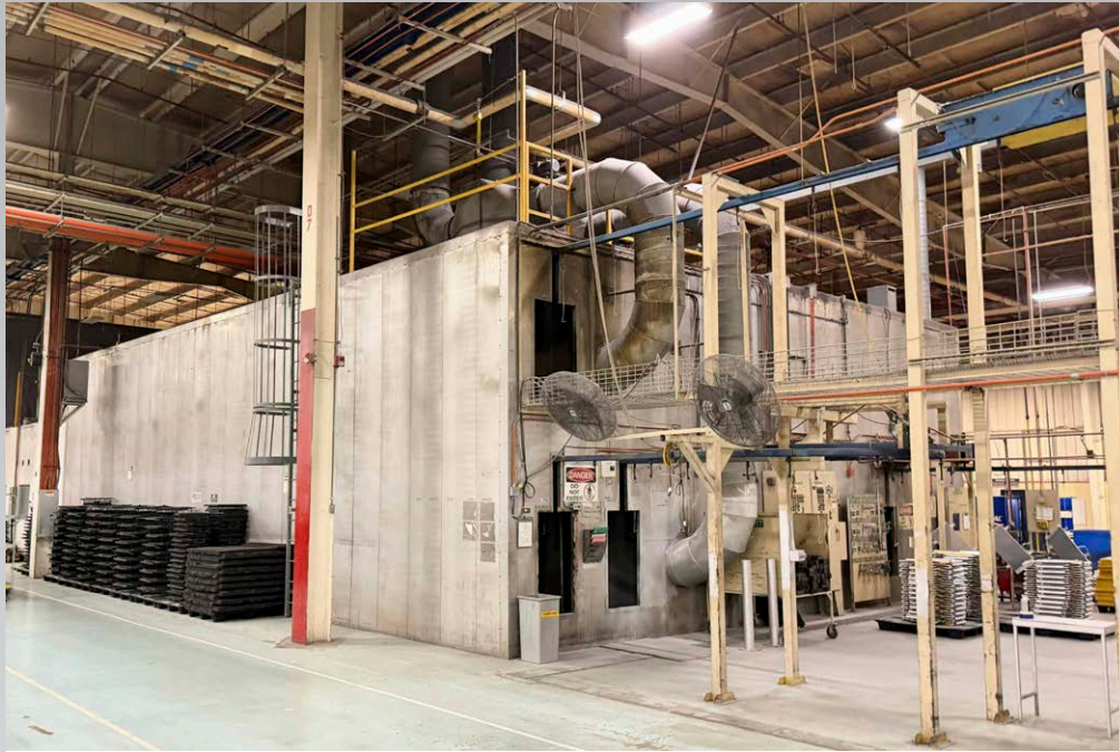
Ionics Paint Booth - Curing Oven - Dry Off
