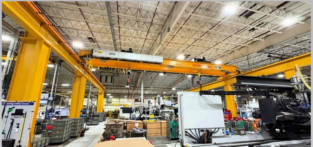
25-Ton Konecranes Freestanding Bridge Crane System
