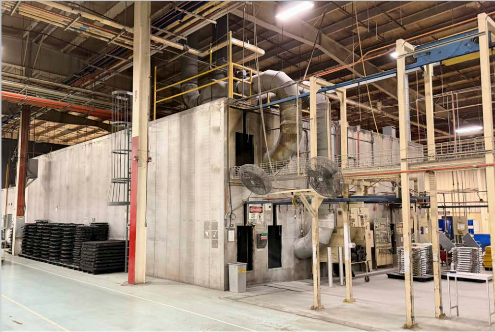
Ionics Paint Booth - Curing Oven - Dry Off
