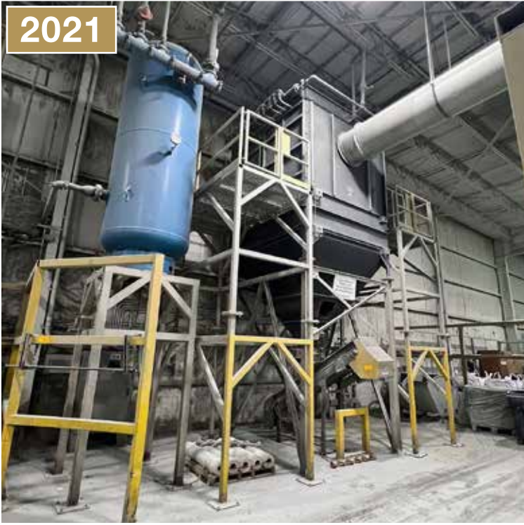
AMTECH Dust Collection System
